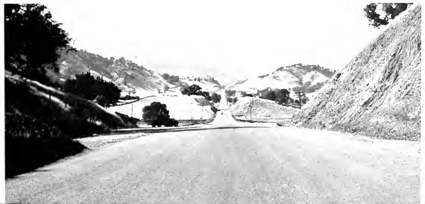
Redwood Highway improvement north of Hopland involved several long deep cuts on new direct routing
